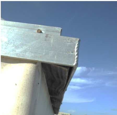
Incorrect measurement will create a gap between the curb and the skylight frame
