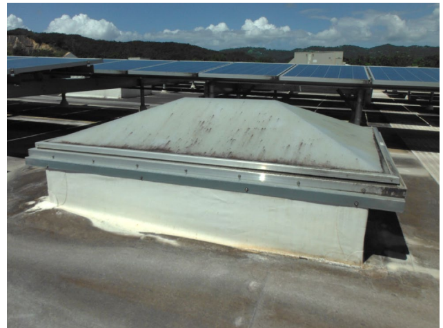
Photo of incorrectly measured custom skylight
