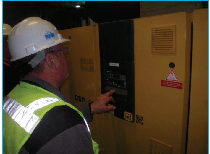
Team reviewing set points on an air compressor. PHOTO COURTESY OF CALPORTLAND COMPANY.
