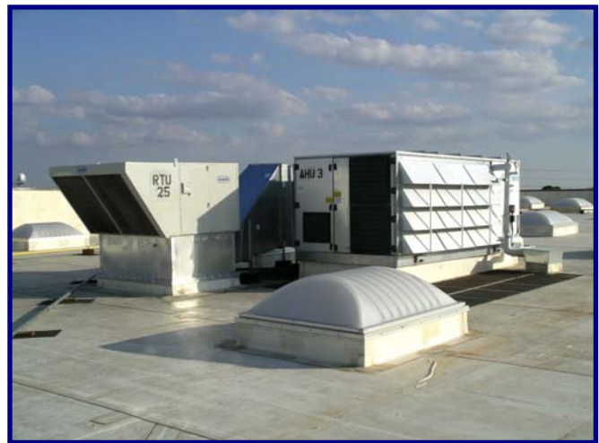
Munters AHU with add-on RTU to left
