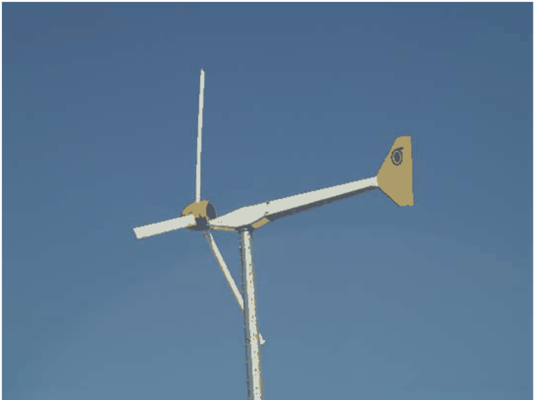
Bergey XL 50 50-kW wind turbine at the center of the site
