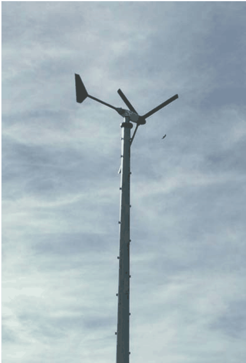
1-kW wind turbine powering the small monument sign at the side entrance
