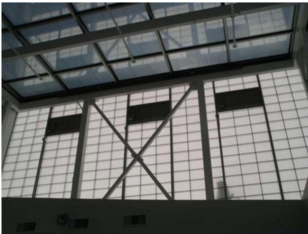
Advanced entry vestibule with thin-film PV glazing roof and translucent upper walls
