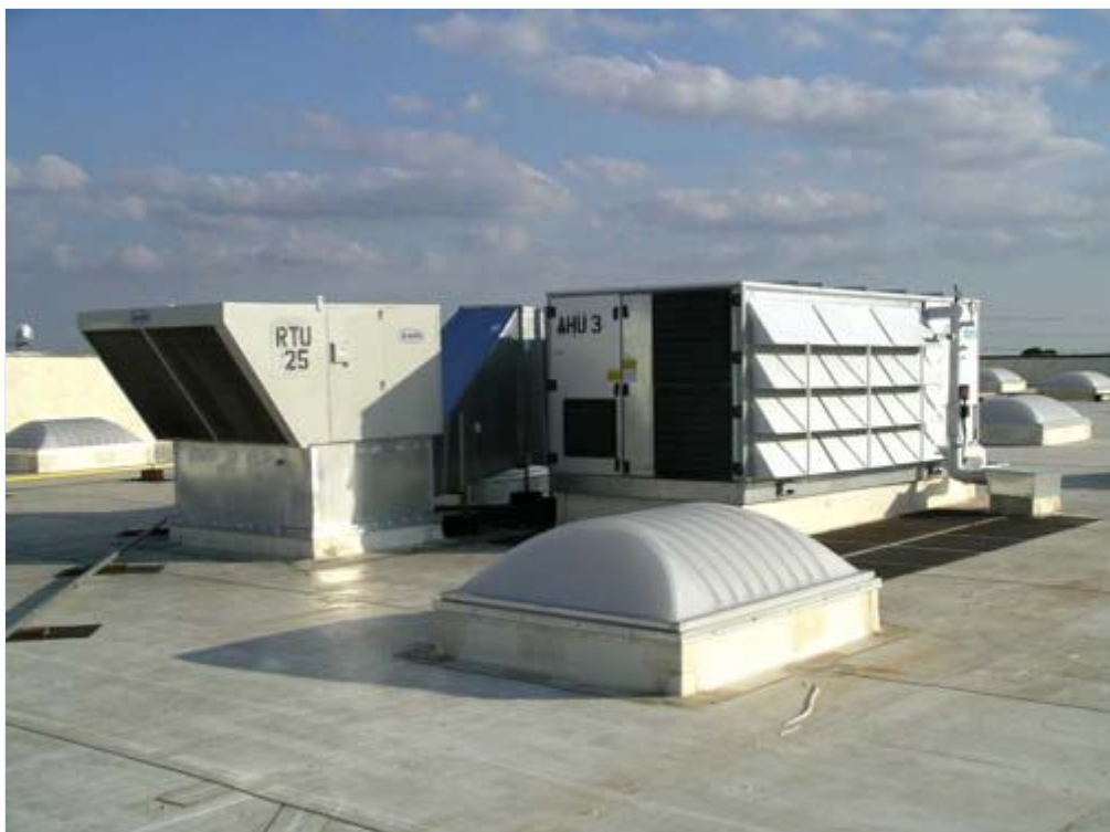
Munters AHU with add-on RTU to left
