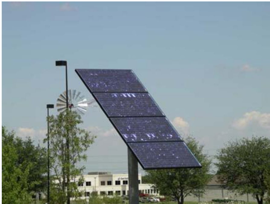
1.6-kW solar PV system for the large monument sign at the main entrance
