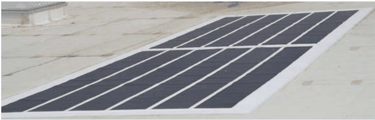
PV Array 3 Sarnafil roofing modules on the auto center roof
