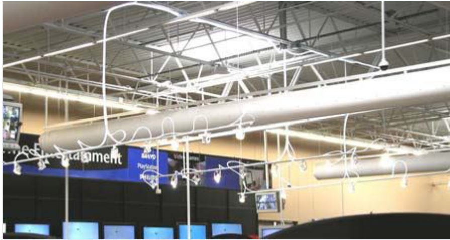
Hybrid Solar Lighting optical fiber ends fixed along a lighting track over the merchandise racks
