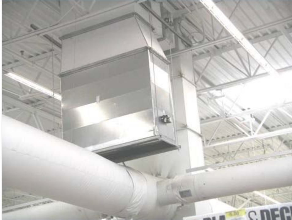
Fabric duct (ductsox) and rooftop unit supply connection above the sales floor
