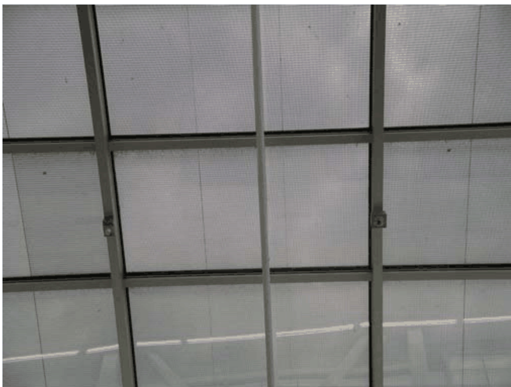
Thin-film PV glazing in the vestibule roof shades direct sunlight while allowing daylight to filter into the space
