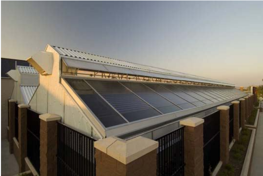
PV Array 4 on the slanted garden center roof
