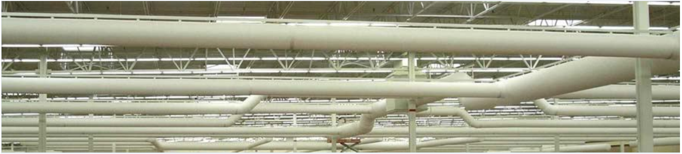
Fabric duct (ductsox) low-velocity thermal displacement air distribution system mounted above the sales floor
